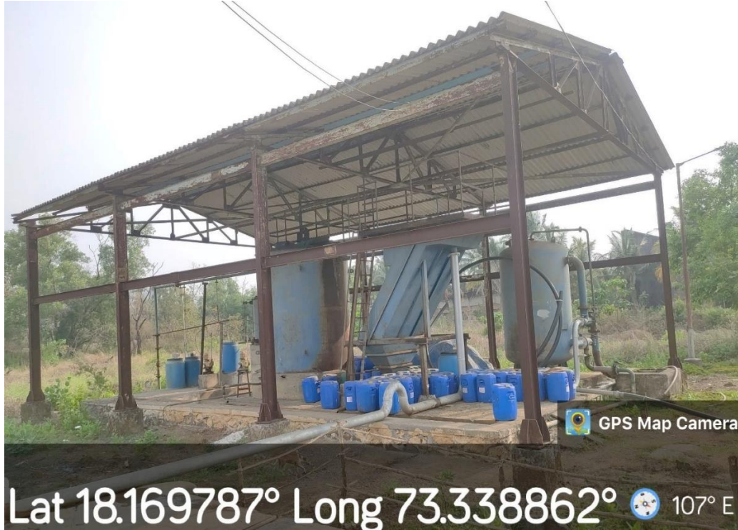
Photos 3 – Water treatment plant near IoPE
