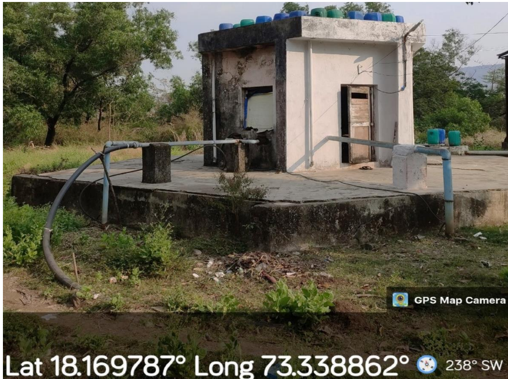
Photo 4 – Pump house near IoPE
