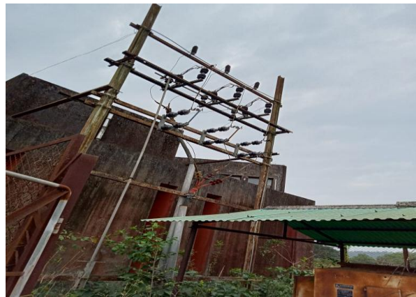
Figure 12: Supply Voltage from MSEDCL
