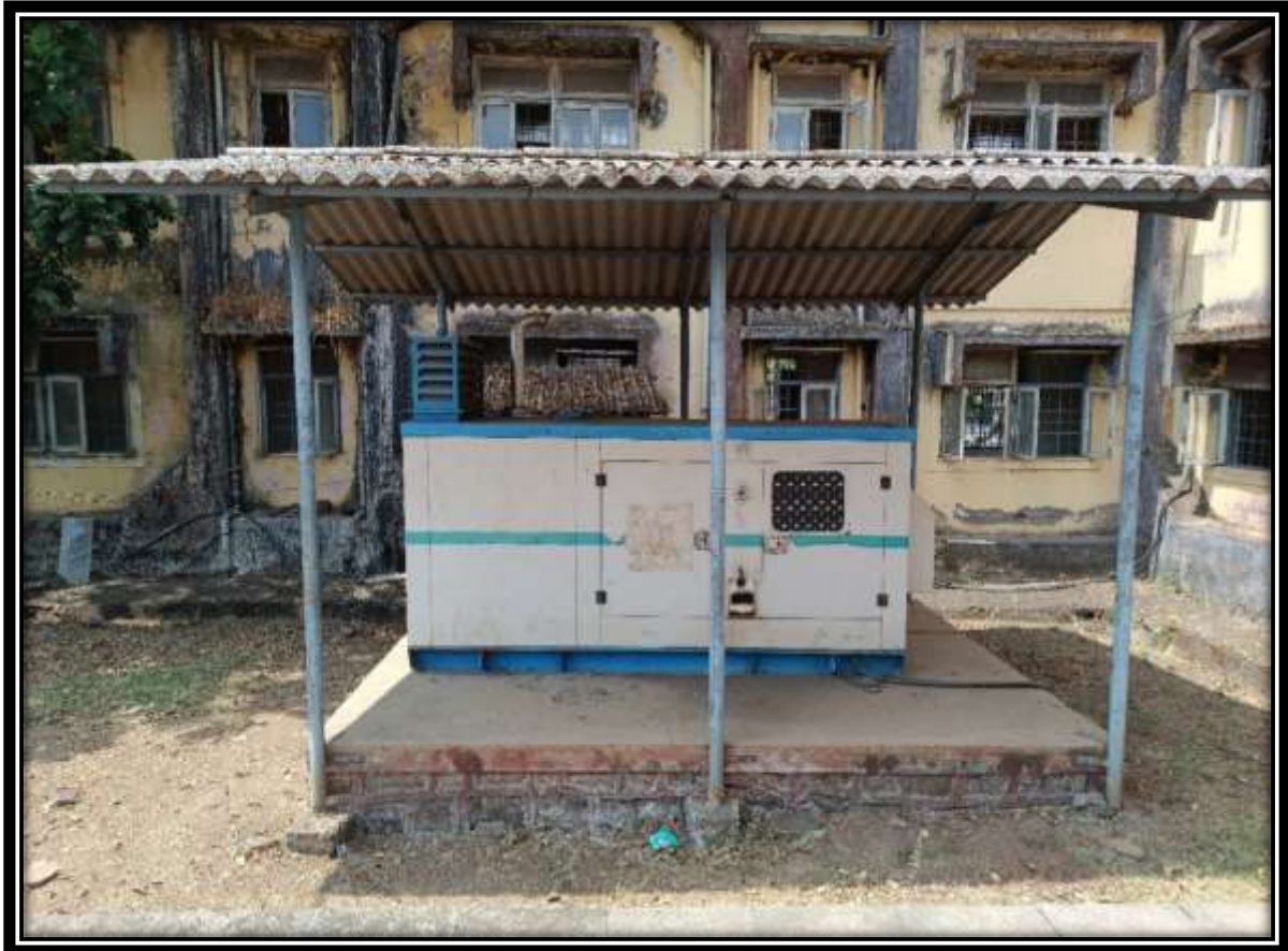
DG Set used for Emergency power supply
