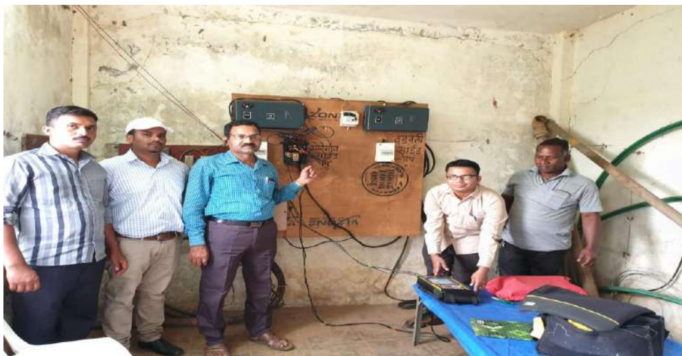
Figure 22: Snapshot of power analyzer reading of Water pump
