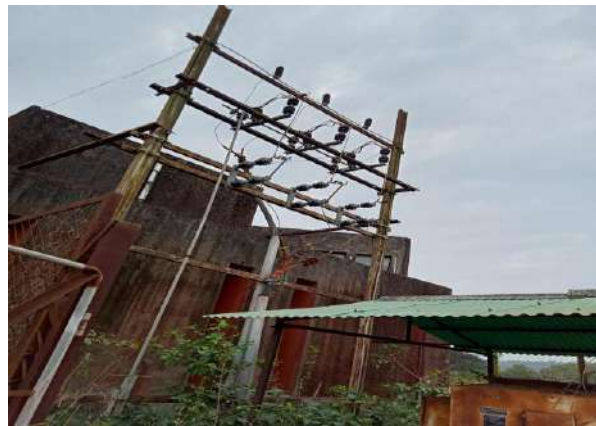
Figure 12: Supply Voltage from MSEDCL
