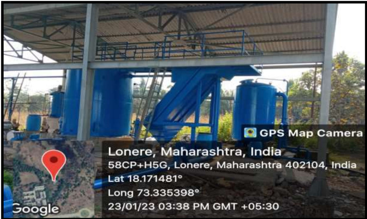
Waste water treatment plant
