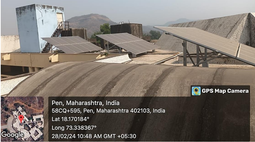
Photo of Solar Panel Installed at Roof top of University Main Building.
