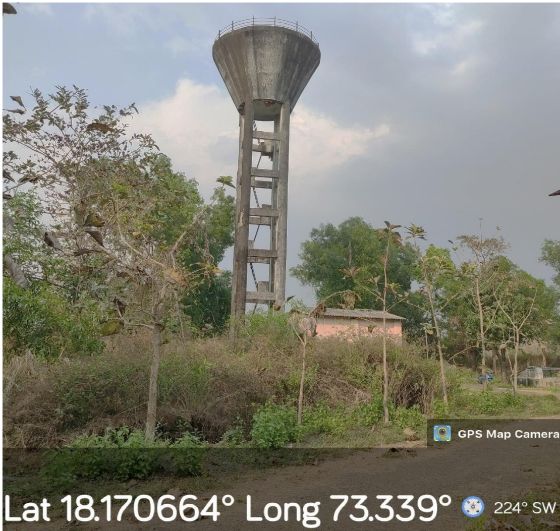
Photo 8 – Water storage tank in University Campus
