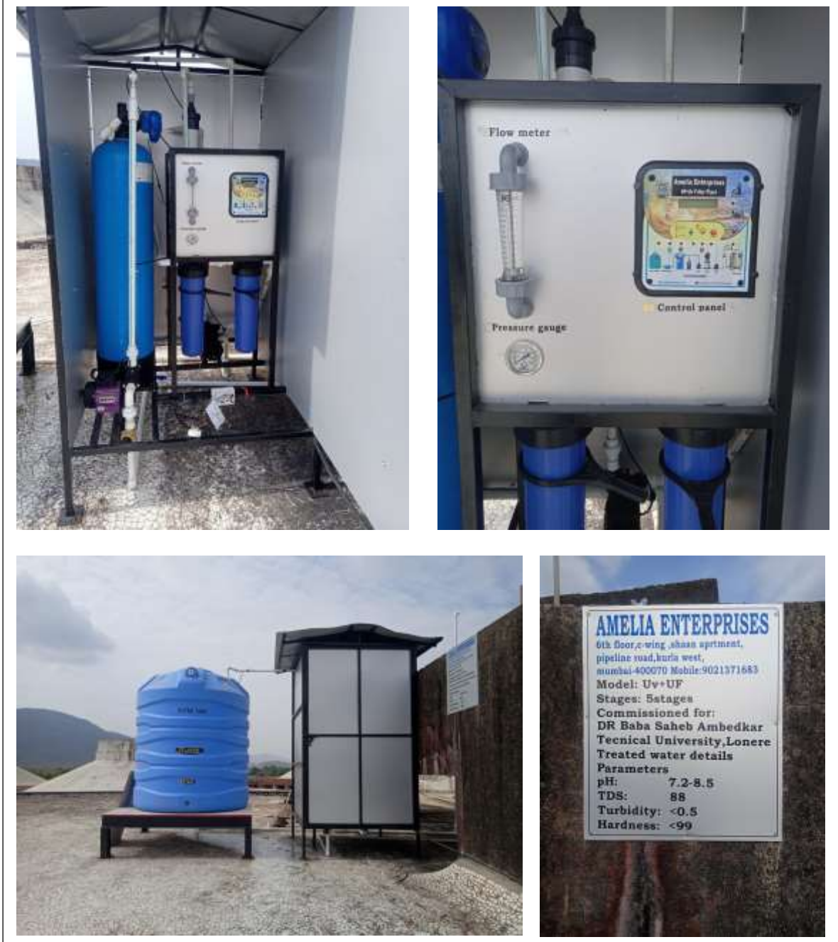
Water treatment facility installed at roof of University building
