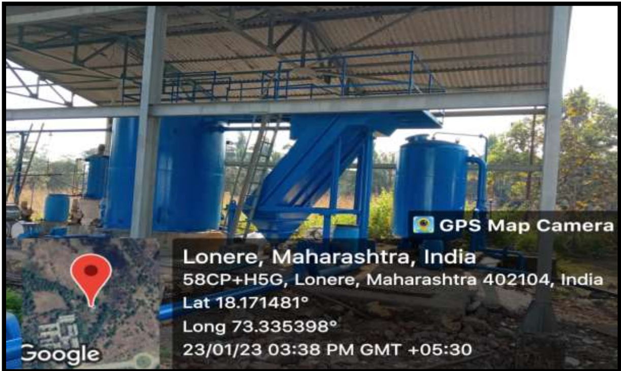
Waste water treatment plant
